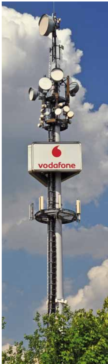
Vodafone OMC tower in Ratingen
